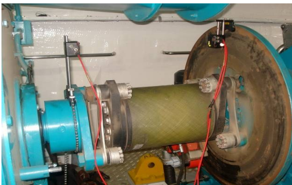
Fig. 8- Drive train alignment in WTG
