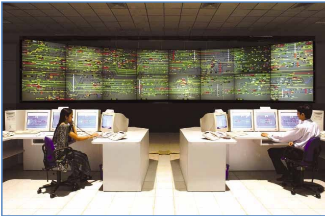
Fig. 3- Video wall with workstations
